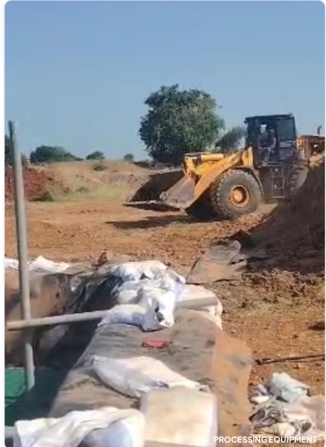
LINED PROCESSING BASIN
